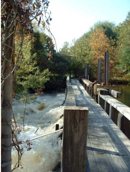
The 173-year-old wooden Whittenton Mill Pond Dam strains to hold back floodwaters.
