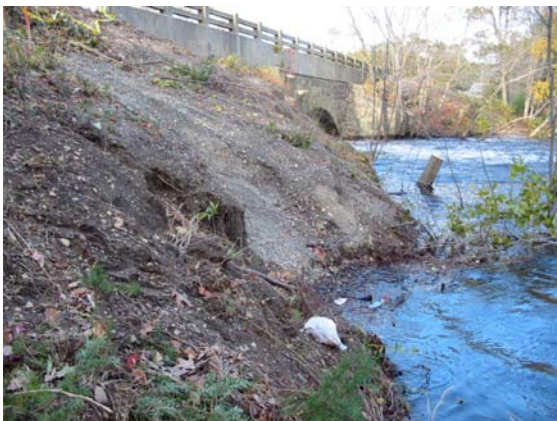
Embankment Erosion, Rice City Pond Dam
